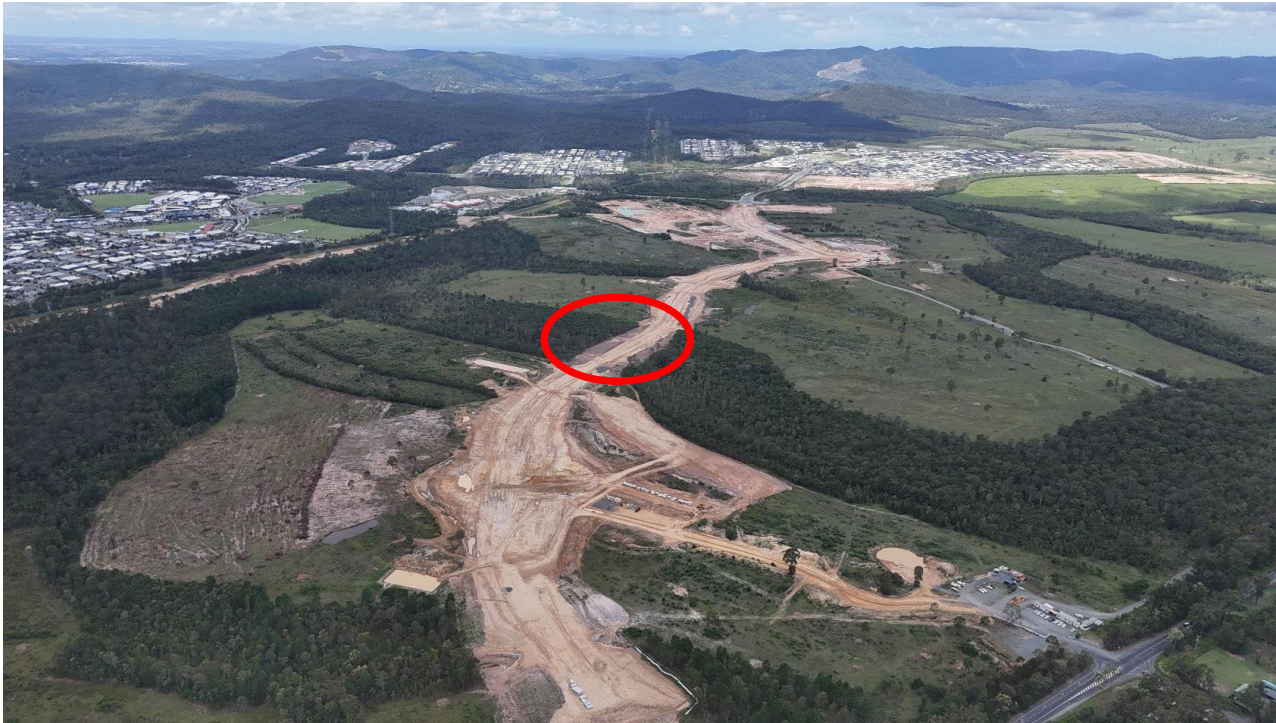
Jimbilunga Drive alignment showing location of new major drainage and fauna culverts
