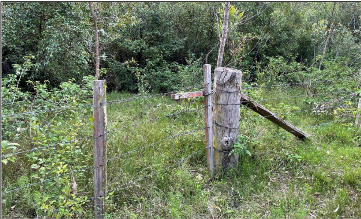
Photo set 2: Before photos - Perimeter fence with top strand of barbed wire
