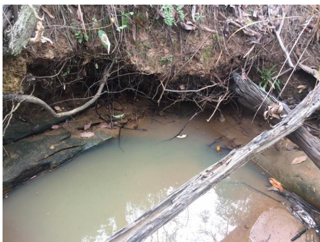
Figure 12: Drainage feature with pooled water
