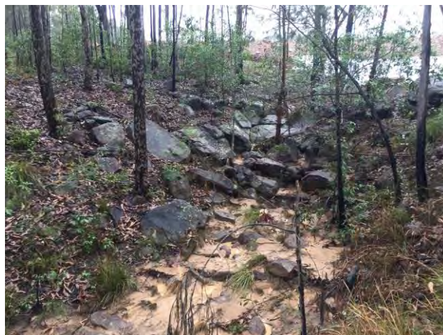
Figure 19: Drainage feature – wet after rain event
