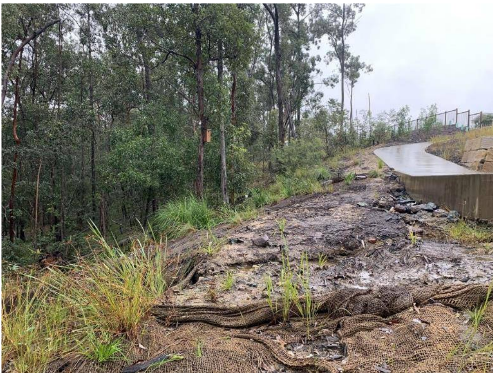
Photo 9: Minor evidence of erosion within rehabilitation area towards the western extent, to be rectified as part of management measures.
