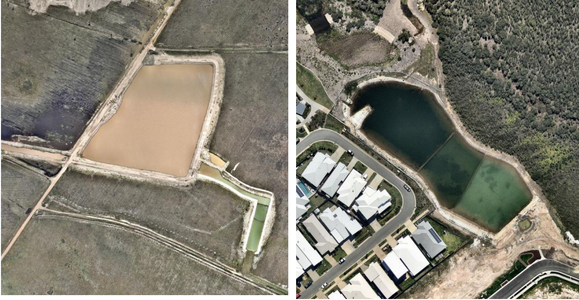
Figure 8: Hybrid Sediments Basins in Operation
