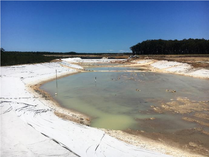
Figure 7: Hybrid Design High Efficiency Sediment Basin with Kidney Shape and Increased Storage Capacity Installed in Precinct 2.
