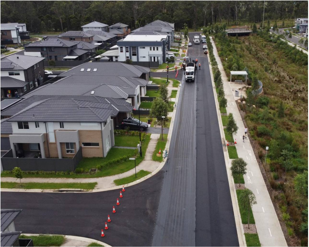
Pics show: Road surfacing in the Elara estate, Marsden Park with Reconophalt.
