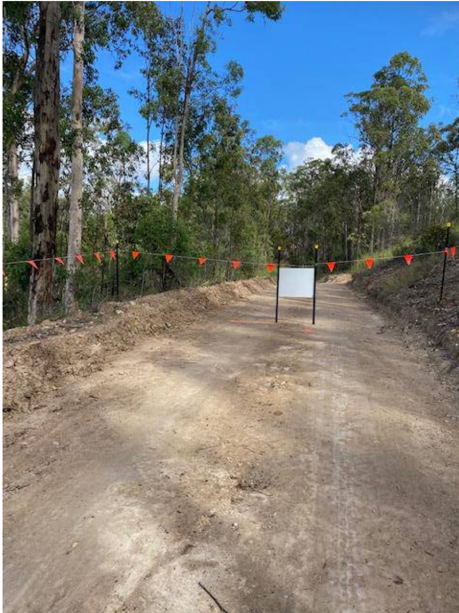
Categorical surveyed demarcation vegetation clearance perimeter fauna friendly fencing was witnessed offering onsite fauna management compliance.
